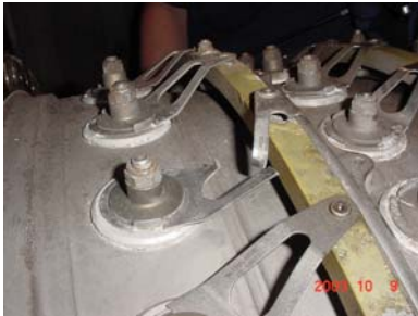
Figure 2-65. Broken VSV caused by Compressor Stall (Stall contributed to lack of proper external waterwash)
