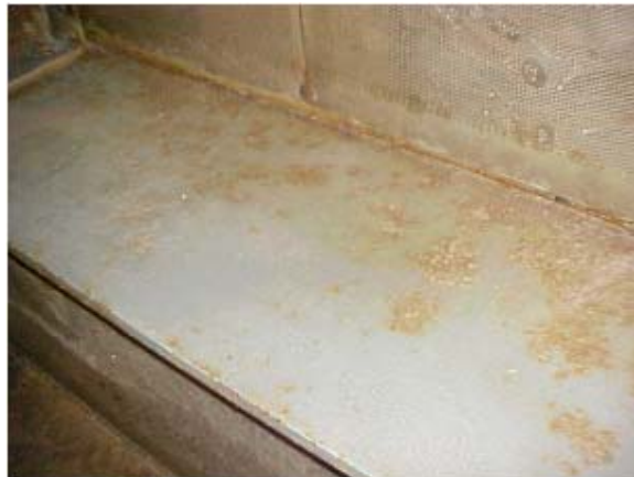
Figure 2-74. Dirty Inlet Plenum
