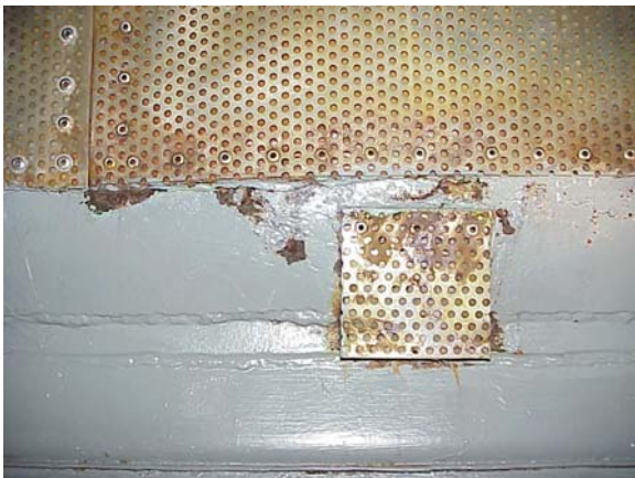
Figure 2-73. Rusted FFG Intake
