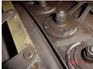
Figure 2-64. Lack of Proper External Waterwash
