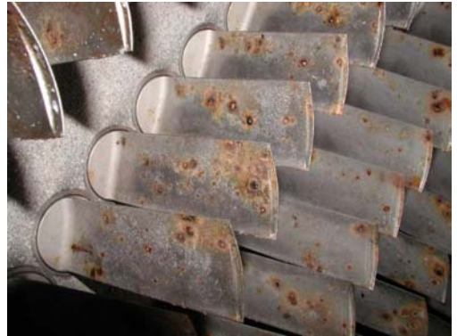
Figure 2-63. Salt and Rust Buildup Due To Lack Of Proper Waterwash
